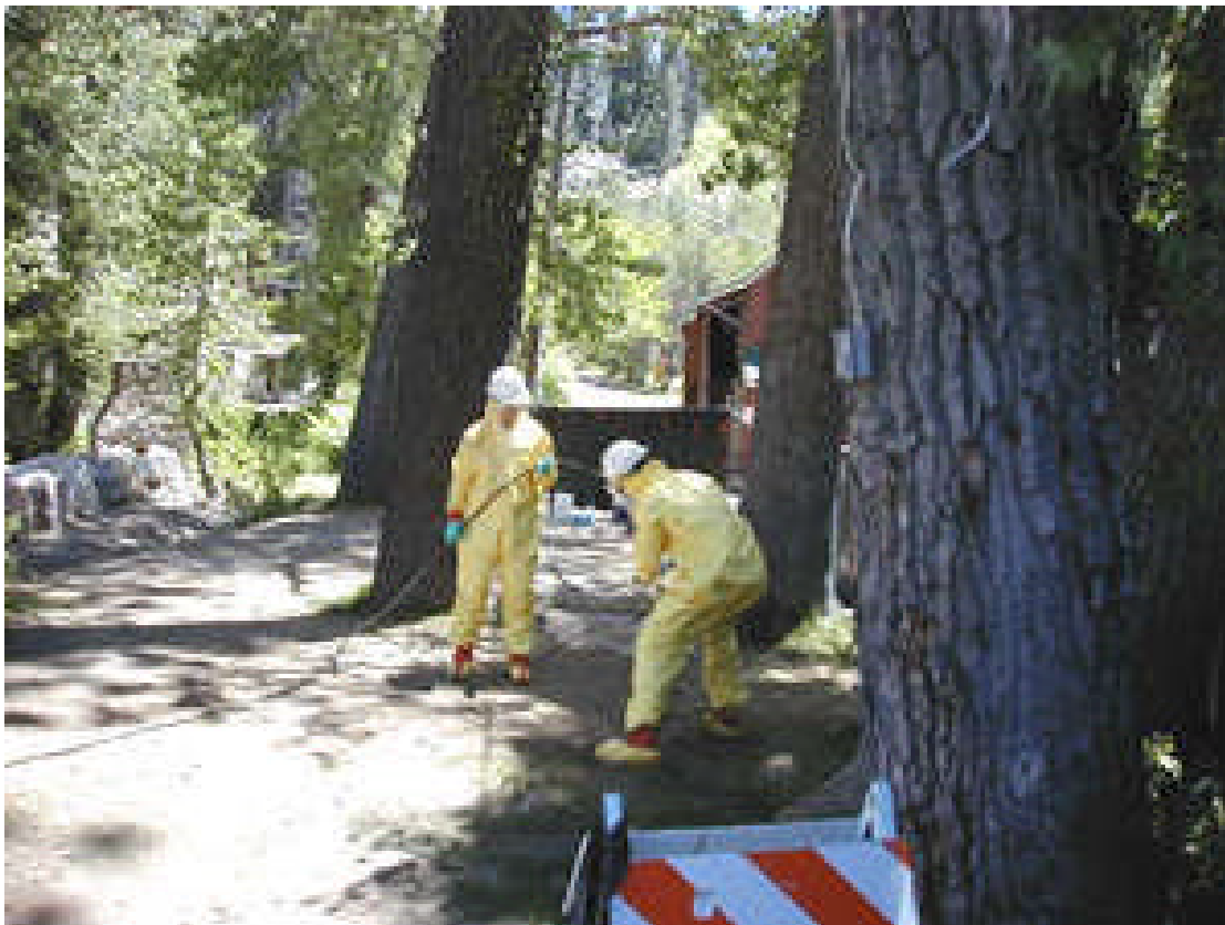
Figure 3 - Jetting using hydrogen peroxide with 12-foot long lances in a limited access environment in northern California (Courtesy FAST-TEK).
