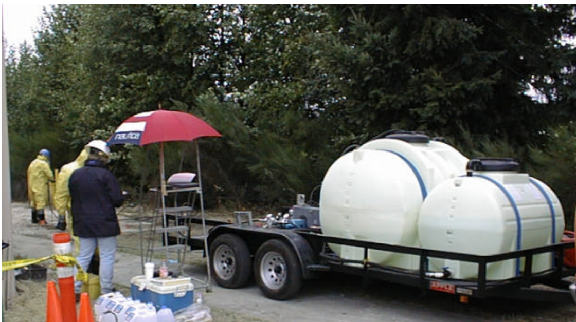
Figure 2 - Injecting hydrogen peroxide on a job site in Tumwater, Washington, (Case 1). (Courtesy FAST-TEK)
