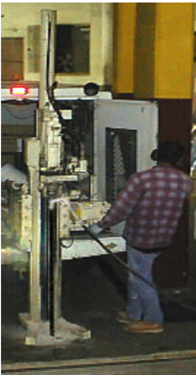
Injecting hydrogen peroxide through the drill rod of a direct push rig.
